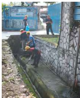
Drainage clearing at the entrance of our factory
