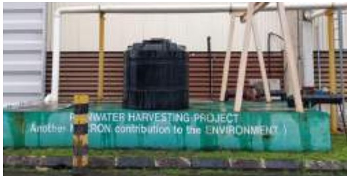
Rainwater Harvesting System at one of the factories
