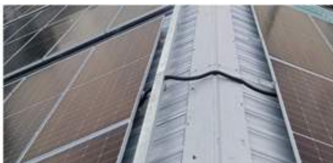
Our roof mounted SOLAR PV system
