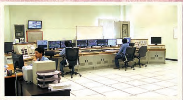
Central Control Room
