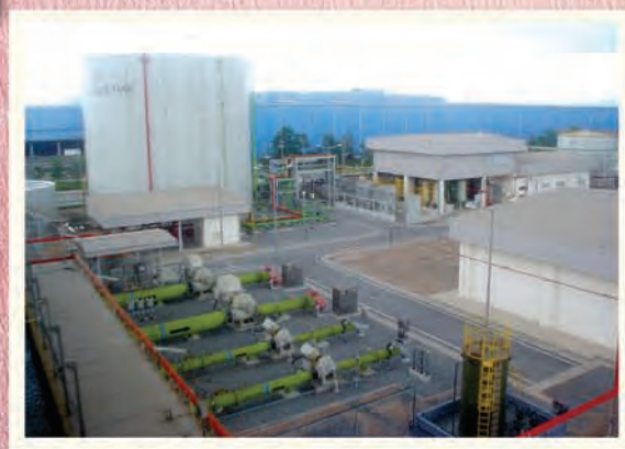
Raw Water Storage System
