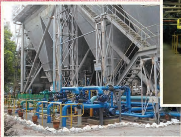
Quenching Water System
