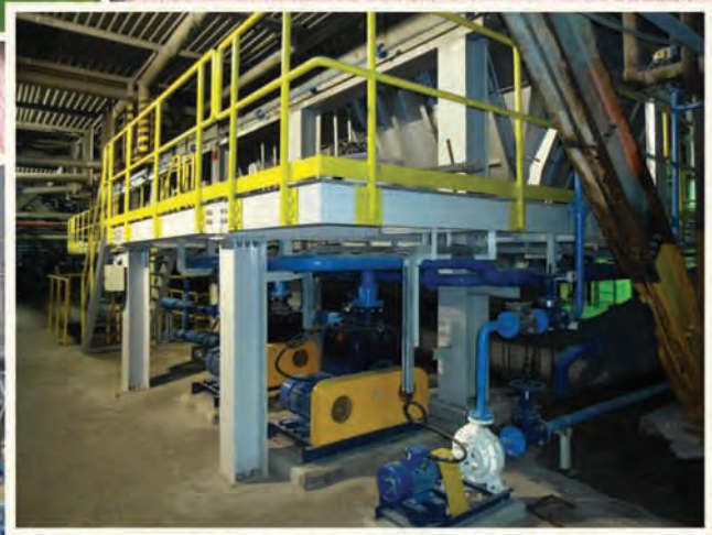
Bottom Ash System – Hopper General View
