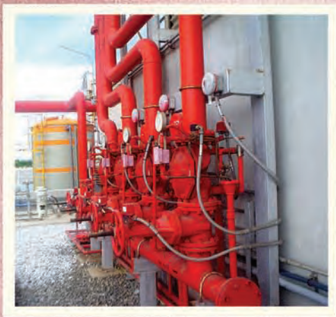
Fire Fighting System
