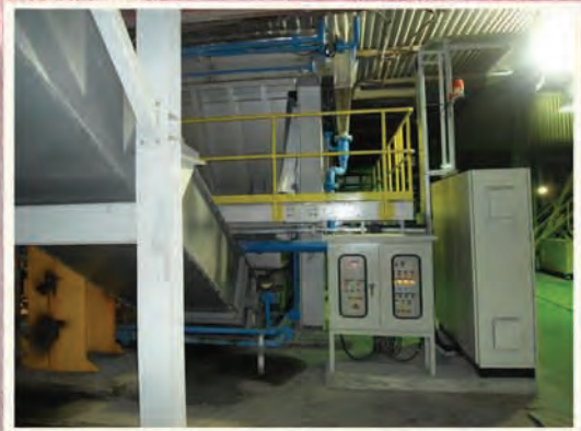
Bottom Ash System – Chain Conveyor
