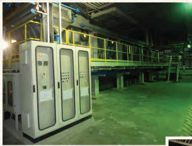
Bottom Ash System – Control Panel
