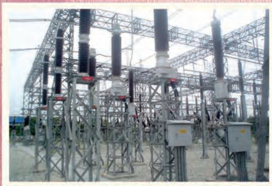
Siam Power's Substation
